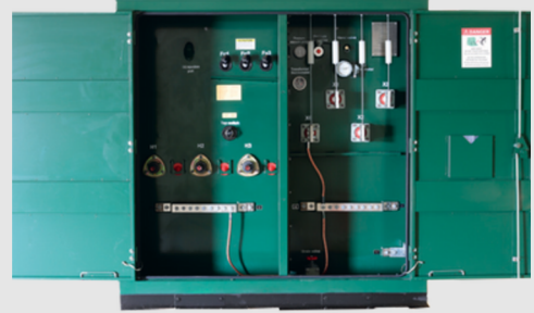
PAD MOUNT TRANSFORMERS
